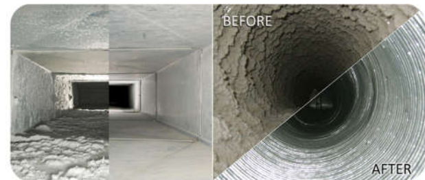
Air Ducting Clean Before & After
