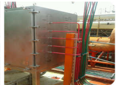
HYDRAULIC VALVE CONTROL SOLENOID BOX JACKET TUBING
